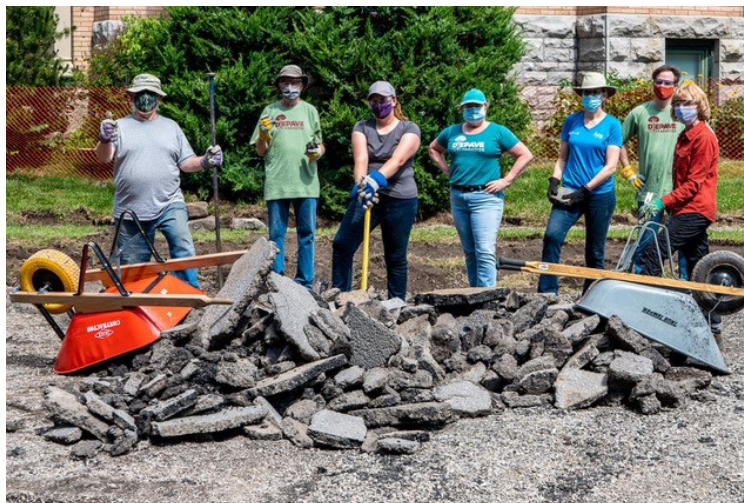
One of the four teams who volunteered to remove a section of Daniel Street on June 19. About one third of that block was removed by hand.
